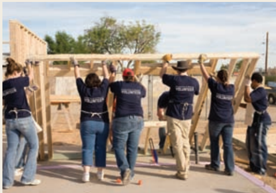
University of Phoenix partners with Habitat for Humanity to build a home for the Jimenez family.
